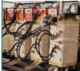
Dry Type Isolation Transformer
