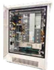
Primary Panel Board
