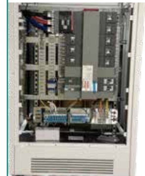
Isolation Transformer & Panelboard
